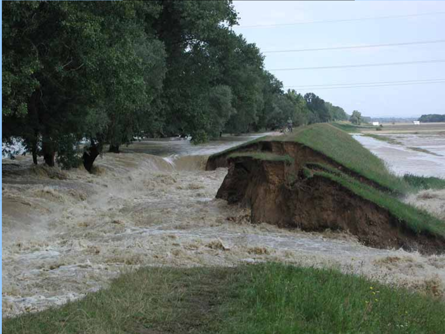
The Ondava River - flood protection dike failure in 2004
