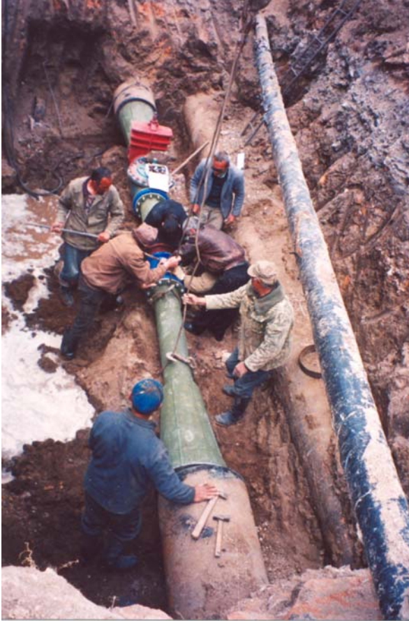
French water engineers using their paid leave to rehabilitate water supply capacities in Gumri, Armenia. This capacity building work is a good example of solidarity between individuals, companies, not-for-profit agencies and local water authorities. Photo credit: Guillaume Aubourg, pS-Eau.
