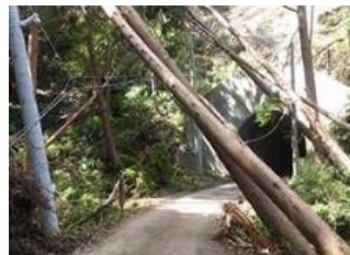
⑨ Collapsing utility poles and trees (Kamogawa-city, Chiba)
