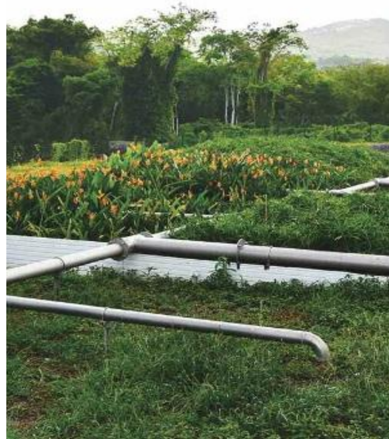
Plant-based water treatment system in Martinique (excerpt from technical guide)
